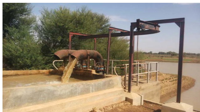
Station de pompage, Mbolo Birane
